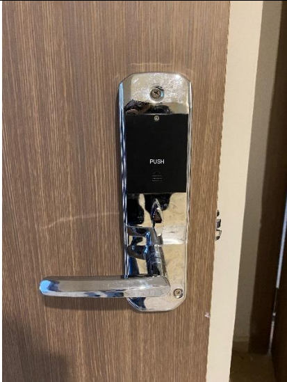
Card System Operated Door
