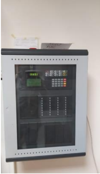
Intelligent Fire Warning System
