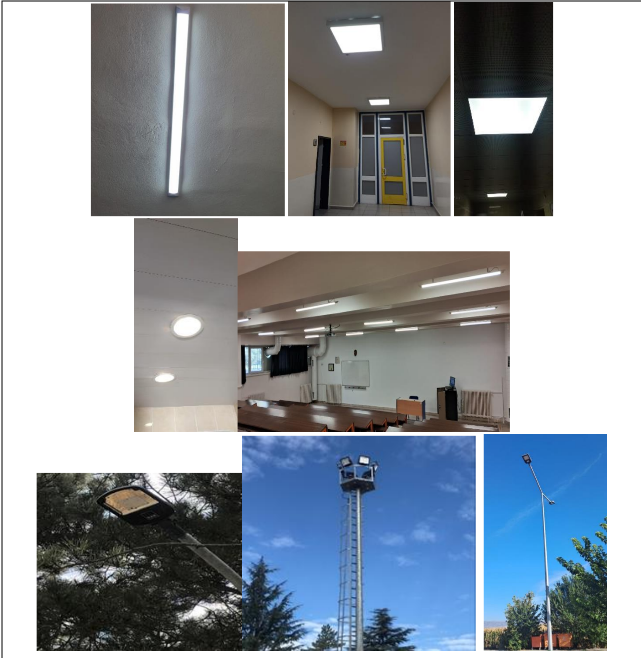
Energy Efficient Appliances Usage: Use of LED lighting and lamps with light detection
